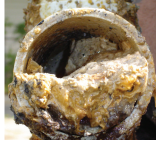
Grease clog inside a pipe.
