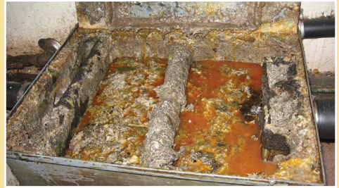
Interceptor too full of FOG and not maintained properly; will cause building sewer problems.
