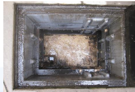
Interceptor operating correctly.
