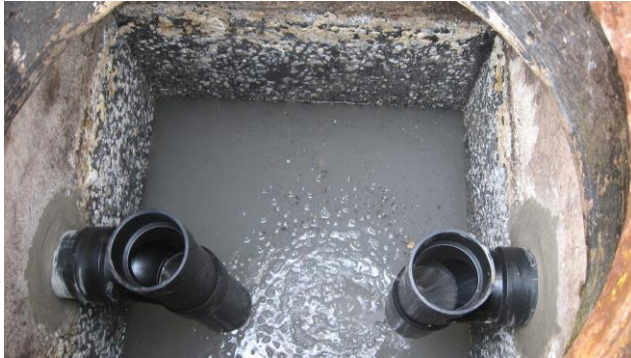
A well-cleaned and compliant grease interceptor.
