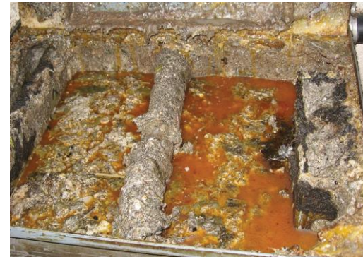
Interceptor pumped out - NOT cleaned to standards.
