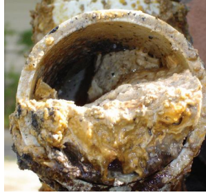
Grease clog inside a pipe.
