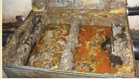
Interceptor too full of FOG and not maintained properly; will cause building sewer problems.
