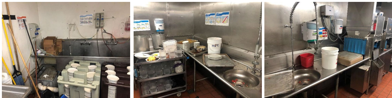
Figure 4: HGI Connected to Sinks, Pre-rinse Connected to Sanitary
